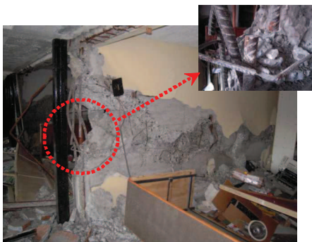
Photo 1 Damage of multi-story bearing wall without boundary columns at the 2010 Chile Earthquake (Tani et al. 2011)
