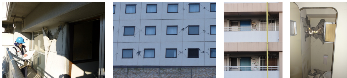
Photo 1 Damage to non-structural walls observed after the 2011 off the Pacific coast of Tohoku earthquake
