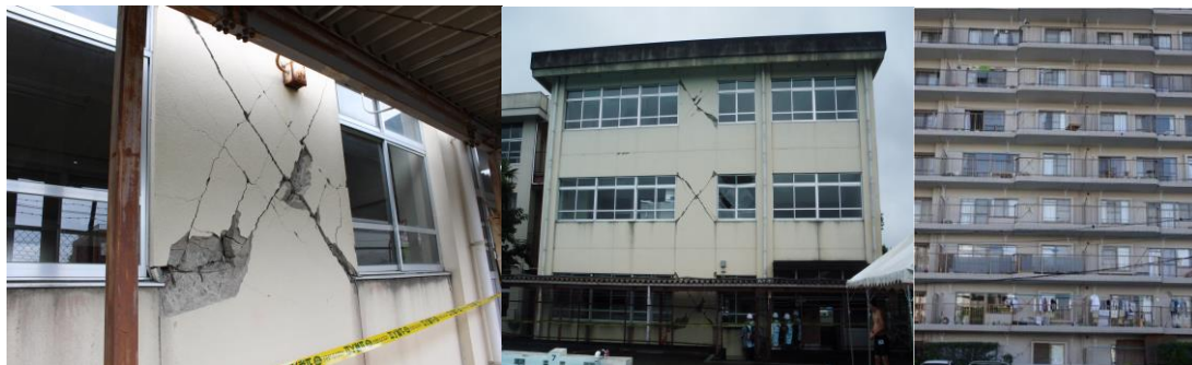
Figure 1 Damage to non-structural walls observed after the 2016 Kumamoto earthquake
